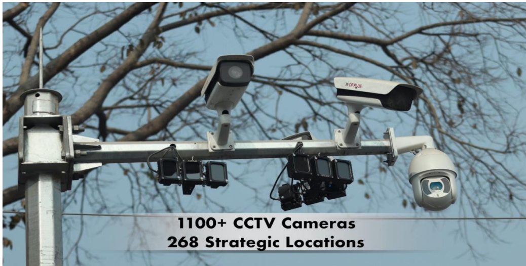
Figure 12.4. CCTV Surveillance System Highlights
